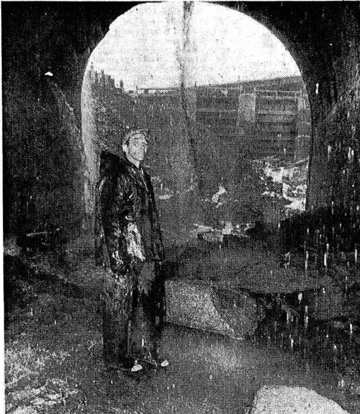
EXPLORER —Richard Waidelich, an employe of the Scufari Construction Co., Tuesday ventured 250 feet into the Schoellkopf power tunnel. He found the concrete liner badly
